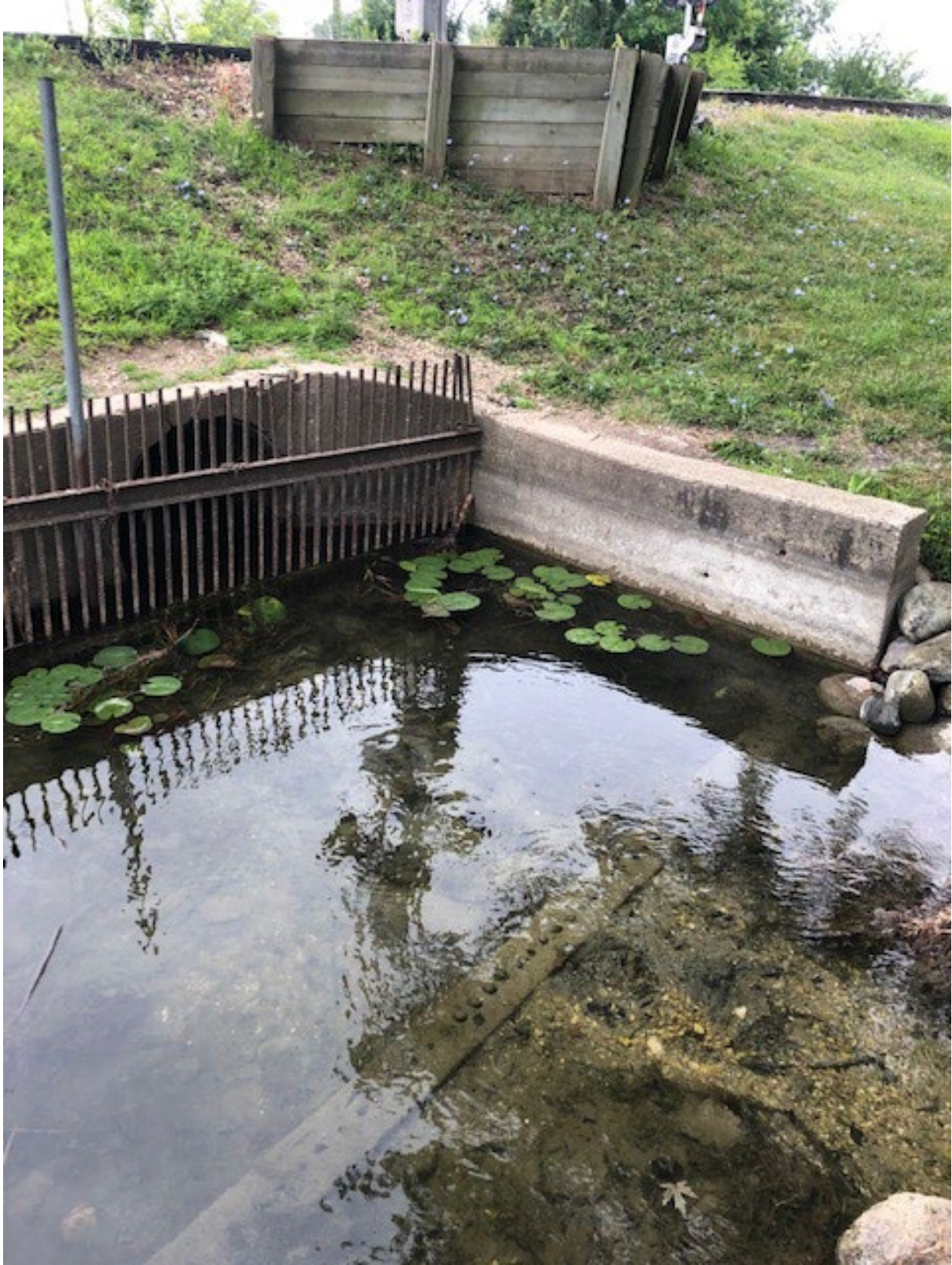
Outlet Creek Culvert Under Silver Lake Road. Note the "summer" water level.
